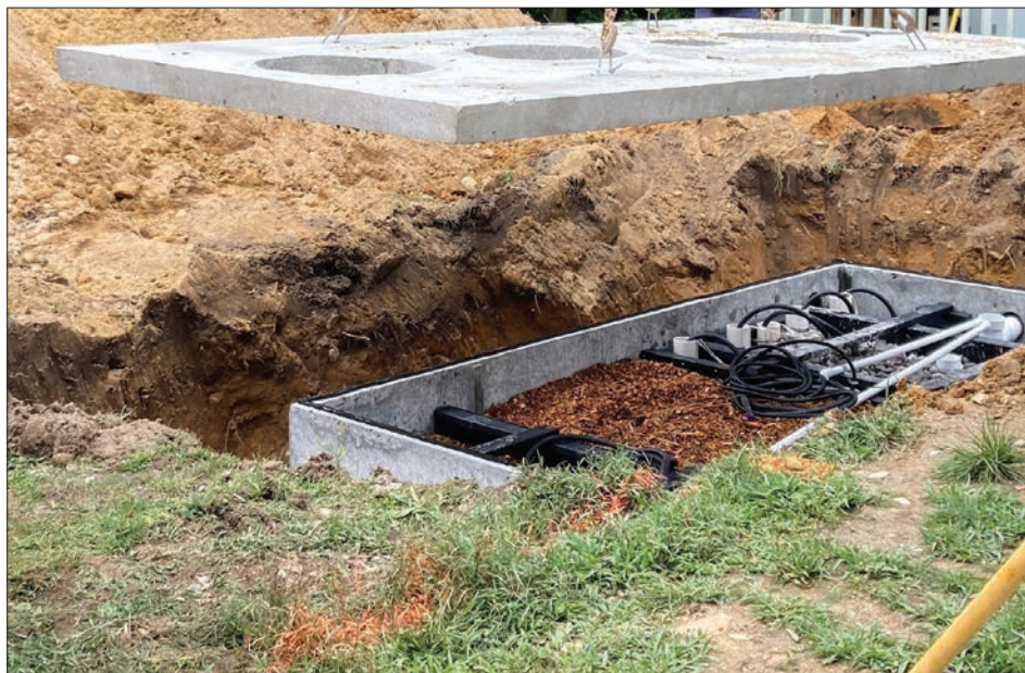
Photo 1. Installation of a NitROE Waste-Water Treatment System with woodchip bioreactor in a neighborhood-scale demonstration study in Cape Cod, Massachusetts. Photo courtesy of Dr. Laura Erban, U.S. Environmental Protection Agency.
