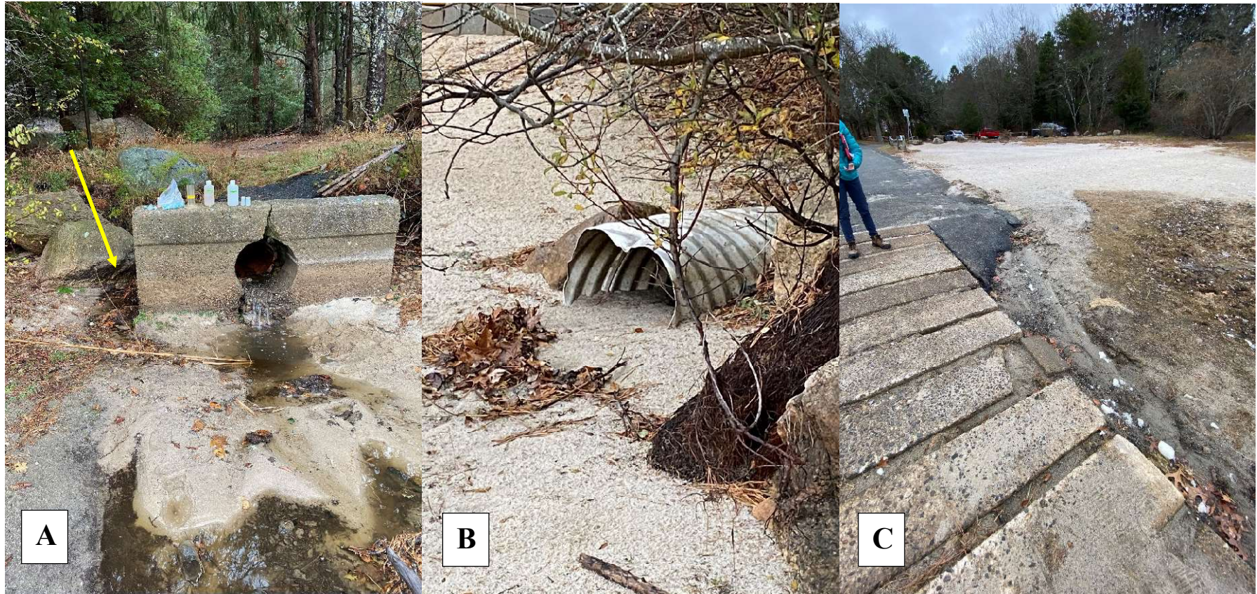
Figure IV-29. Direct Stormwater Runoff Discharge Locations to Shubael Pond. Stormwater discharges to Shubael Pond at three locations: A) a headwall pipe at the end of Shubael Pond Road, B) a corrugated aluminum pipe approximated 5 m to the west of the headwall and C) the boat ramp at end of Willimantic Drive. Based on monitoring during three storms, the largest source of stormwater runoff and nutrient loads is the headwall pipe, which is connected to a series of catch basins on Race Lane and Osterville West Barnstable Road (~0.5 km to the north). The corrugated aluminum pipe is connected to a series of catch basins at the eastern end of Evergreen Road. The boat ramp receives runoff from a portion of Willimantic Drive south of its intersection with Mansfield Avenue. During the two larger storms, a small amount of stormwater flowed directly from Shubael Pond Road, which is unpaved, around the headwall (yellow arrow in A) and discharged into the pond.
